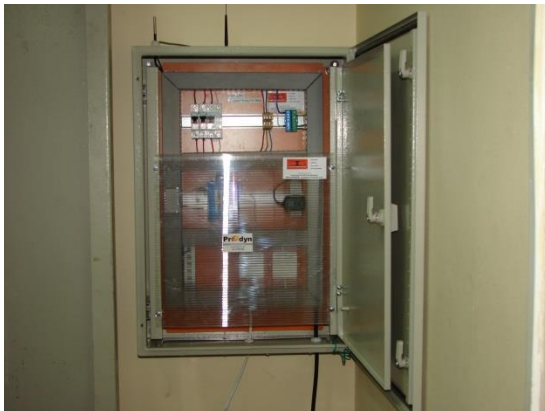
Box containing data devices.
